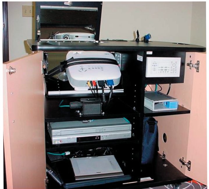
Inside view of an AV cart. The projector throws a reverse image onto a mirror, which bounces to the classroom screen. The SP Controls PixiePro panel, which controls all of the equipment in the cart, is to the right of the projector.
